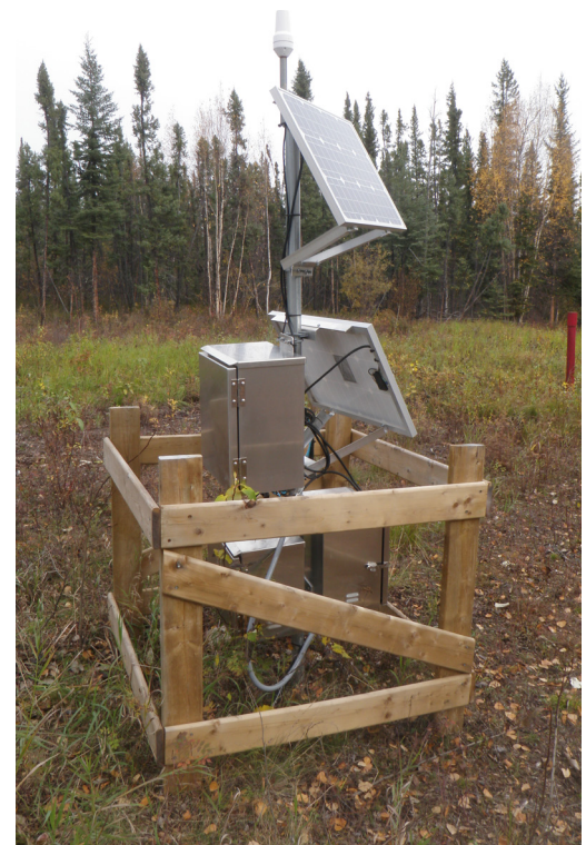
An Enbridge earth station with solar panels, batteries, a data logger and antenna. Earth stations are used in remote areas to power slope monitoring instruments which measure and record ground movement.
