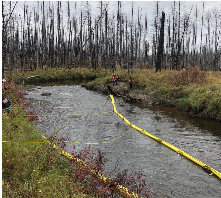
Figure 2-1. Example of a river containment boom in the process of being set up (Enbridge, 2022a).
