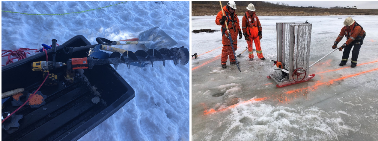
Figure 2-5 Winter response equipment and tactics including an ice auger (left) used to locate subsurface oil and a sled-mounted chainsaw (right) that is used to slot ice (Enbridge, 2022a).
